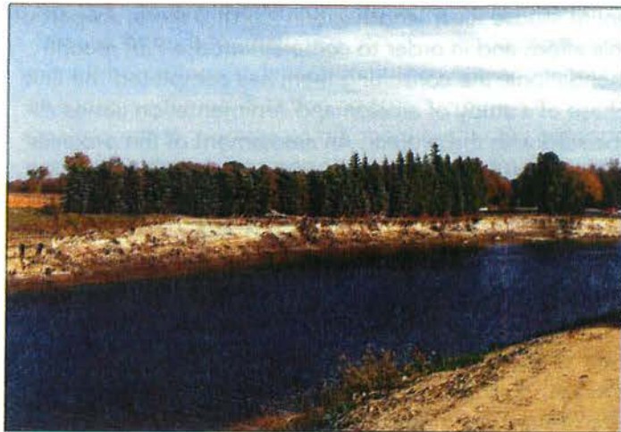
Figure 1: Significant erosion downstream of the Highway 41 bridge at Velva is illustrated by the proximity of the pine trees to the riverbank—before the 2011 flood, about 300 feet of land stood between these trees and the river
