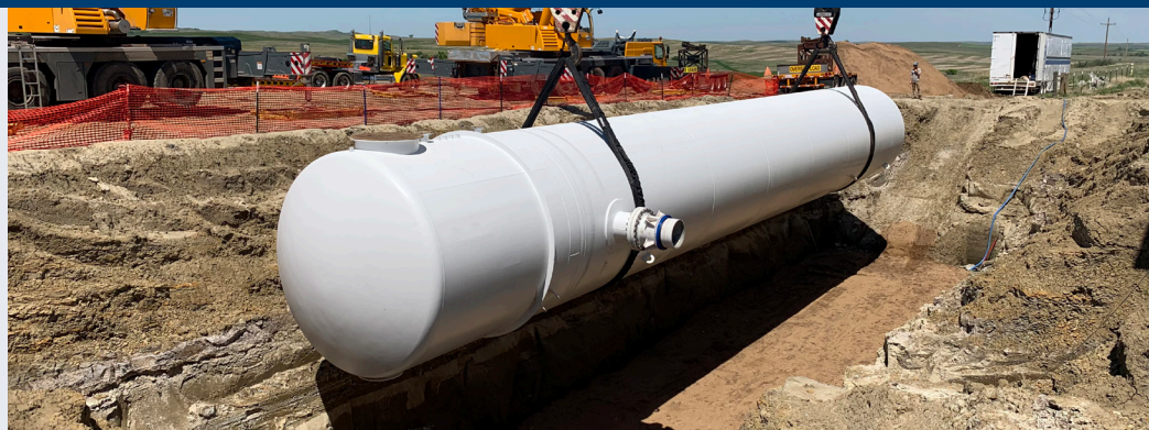
During the 2021 field work season, two new air chambers were installed at the Richardton Pump Station. These upgrades will help increase the raw water transmission capacity.
