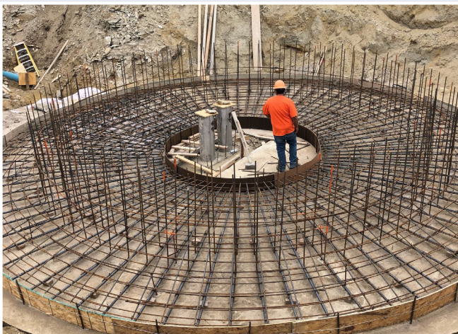
Concrete is poured at the elevated tank in Taylor, ND. The tank is a strategic improvement project to address a waiting list in the Davis Buttes service area.
